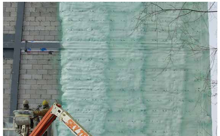
Heatlok Soya HFO being installed directly on CMU block from the exterior.
