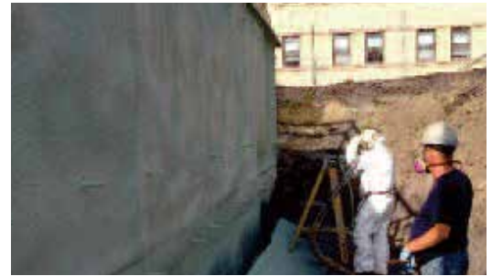
Drainage membrane that will be lifted in front of the foam as the soil is backfilled.
